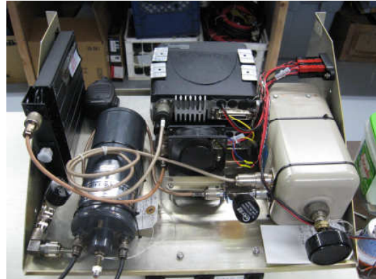
440 Mhz link to Gunderson from Striped Peak equipment shelf under test.
