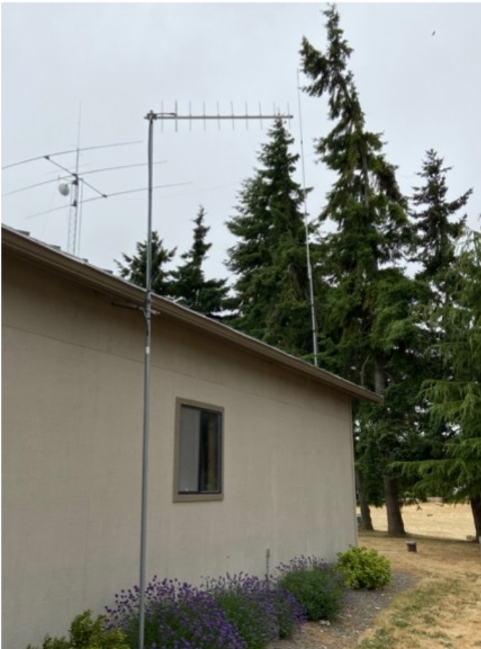
UHF Yagi on 20 foot mast White VHF antenna in front of trees
